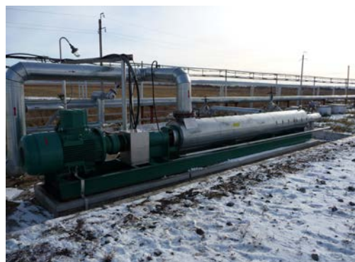
Figure 24: Electrical trace heating and lagging keep the elastomer warm.
