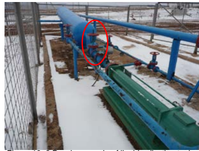
Figure 19: 2. Russia example of liquid collection tank and back flow line and manual valve
