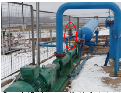
Figure 18: 1. Russia example of liquid collection tank and back flow line and manual valve
