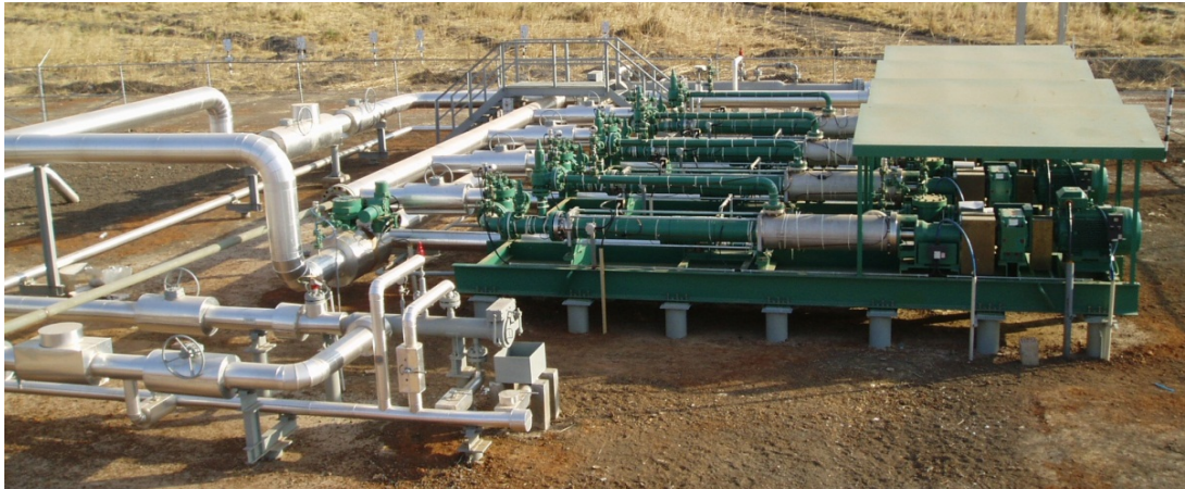
Figure 26: Pump in Sudan working since 2005. Sunshades protect critical equipment from direct sun and high black body temperatures.
