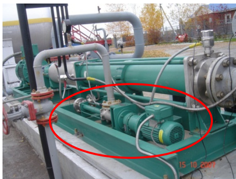
Figure 16: Multiphase pump with small lubrication injection pump
